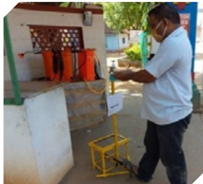
New Taps were installed with hand sanitizers at entry and exit gate @ GHCL Manaparai. Unit
